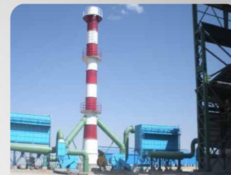
Fume Extraction System
